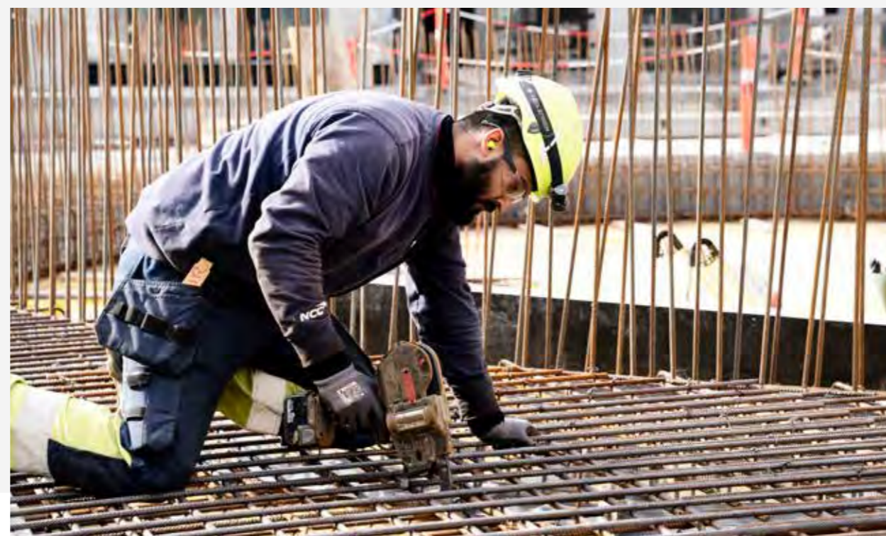
Sammir - a member of PensionDanmark - working on a reinforcement project for NCC.
