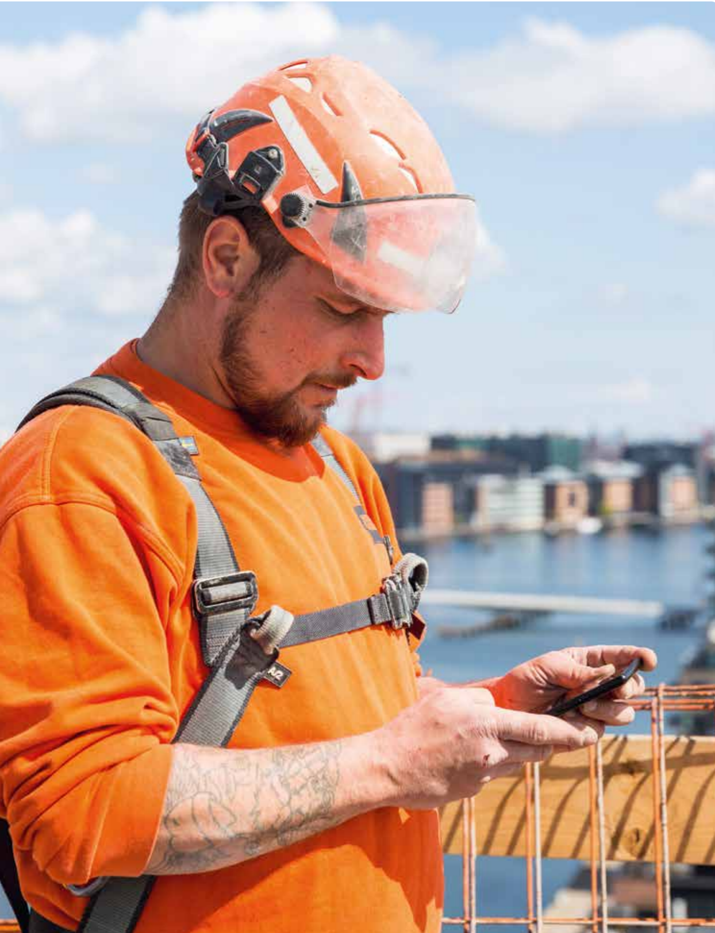
Brian works at Sirius, PensionDanmark's construction site at Islands Brygge and is a member of PensionDanmark
